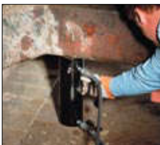
◀ A RAR-506 was easy to position under a bulldozer for repair of frame member.
